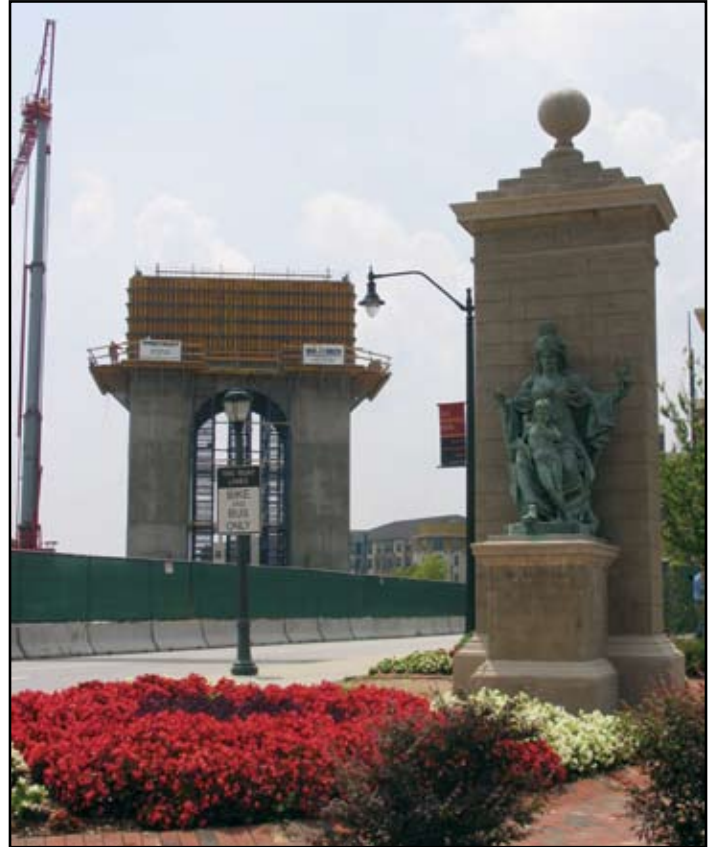
Construction on the $18-million monument, originally planned for Washington D.C., officially began in 2005.
